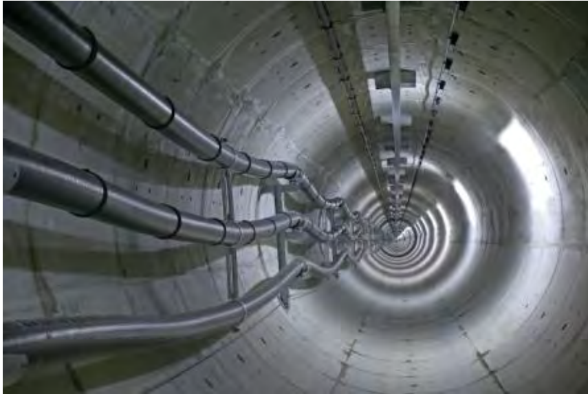
Figure 5.5: Cables running along the side of tunnel (Note: the tunnel illustrated only accommodates 3 cables)
